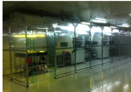
Class 1000 Clean Room
