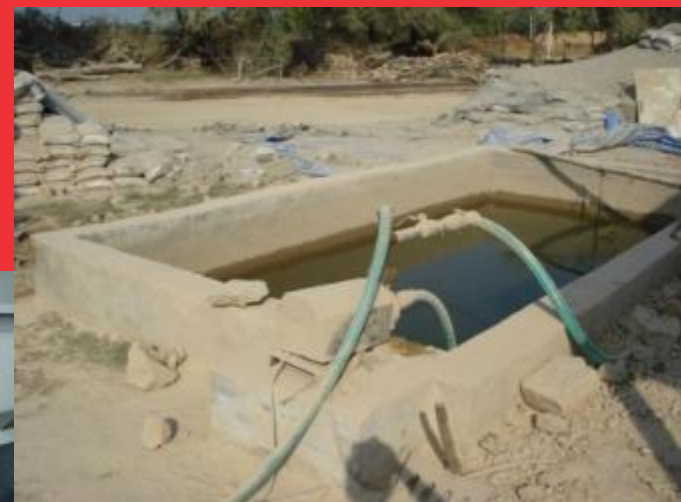
SMALL POND CAN ALSO BE CREATED AS AN OPTION TO WATER TANK
