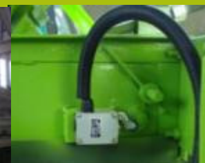
NO FLOW INDICATOR SWITCH
