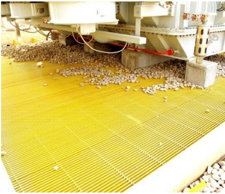
Electric substation flooring
